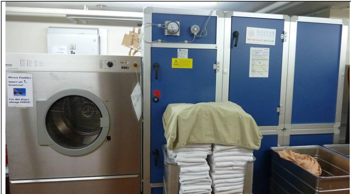
Figure 5.21: A heat recovery system installed in a hostel laundry
