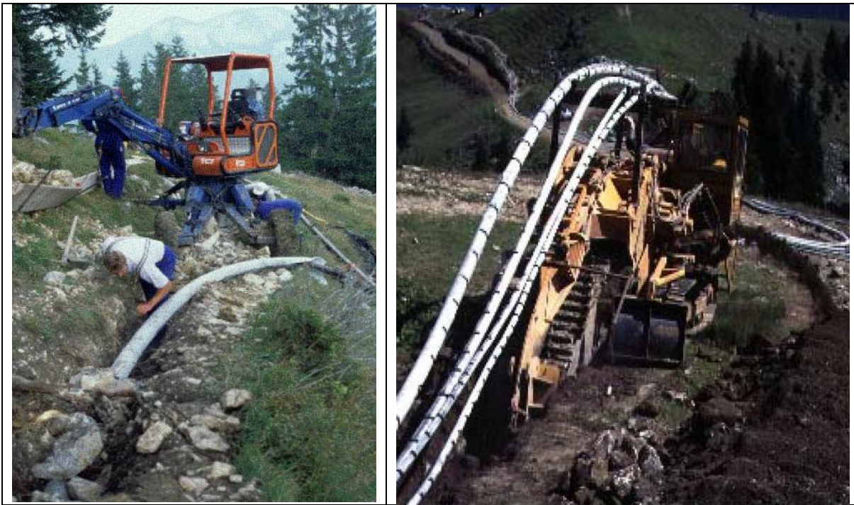
Figure 6.22: Installation of a pipe to discharge wastewater down to the valley to a municipal wastewater treatment plant, (BLU, 2000)
