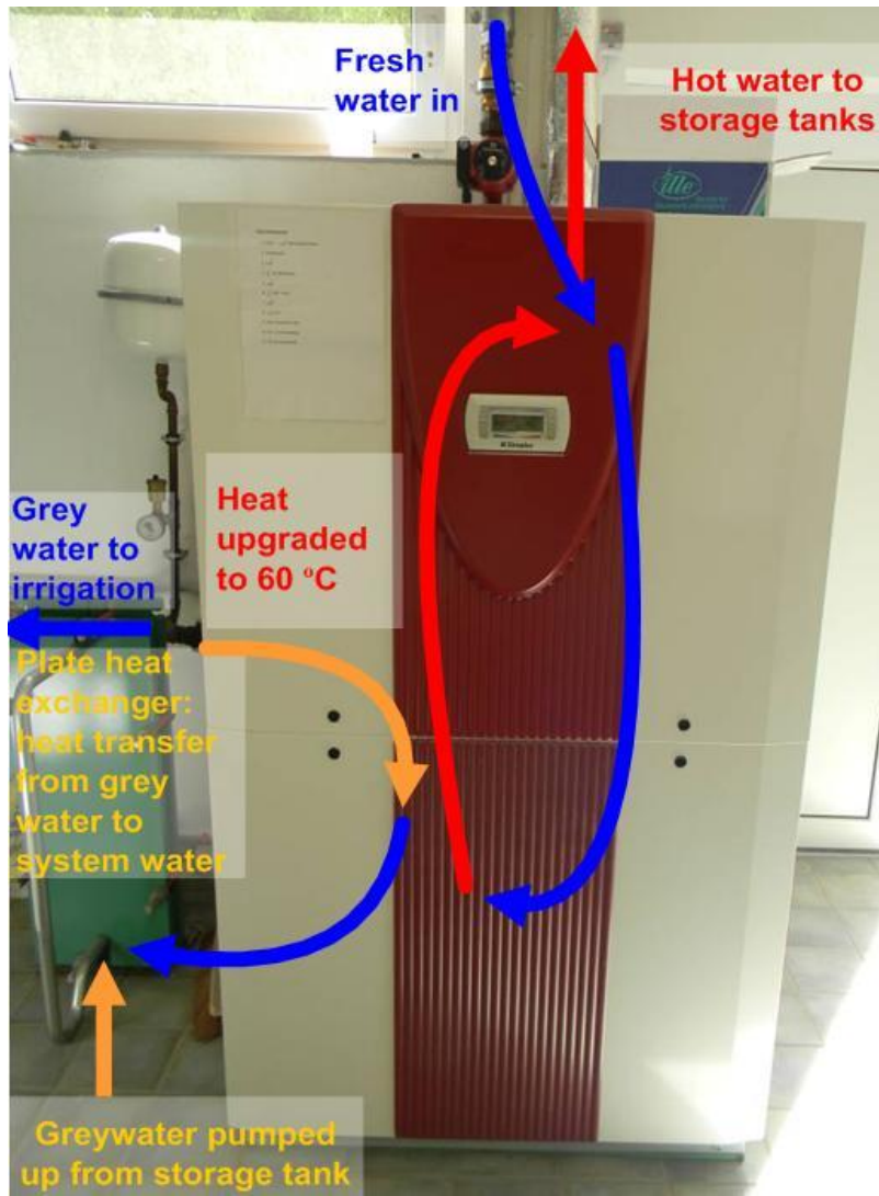
Figure 9.18: Plate heat exchanger (left) and heat pump (centre) used to extract and upgrade heat from washroom and laundry grey water to heat washroom water at Kühlungsborn Camp
